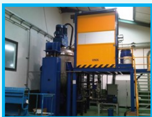
Reactor de grasas (food grade)
